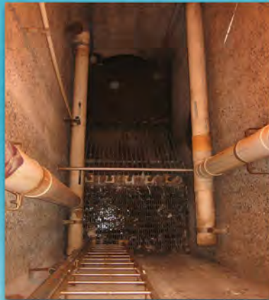
Pump Station before Screentec
