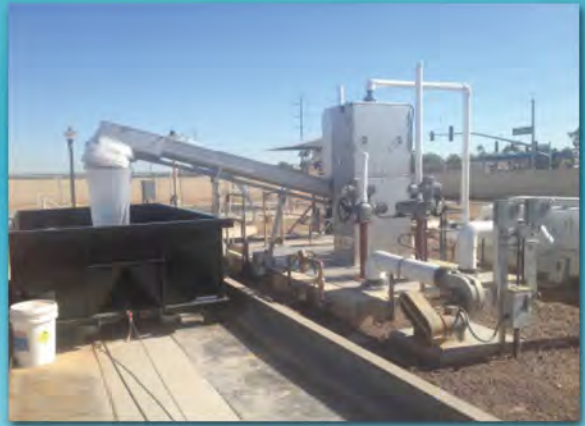
Pump Station with Screentec
